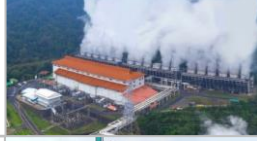
Salak & Darajat Unit 7 40 MW Java, Indonesia
