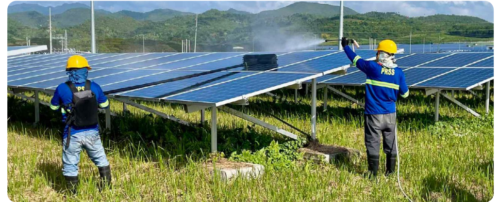
In the Philippines, our 45 MW SaCaSol project uses rotating brushes to clean module surfaces while minimizing water use.
