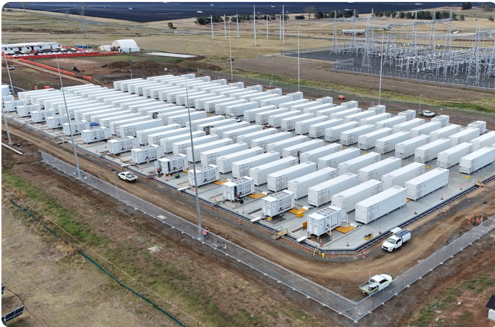
ACEN Australia's 200 MW/2 New England Battery Energy Storage System (BESS) began construction in 2025. It is the first large-scale battery storage project to be built in New England.
