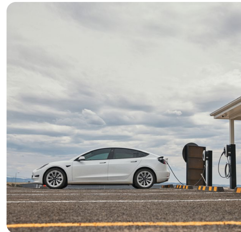
At Stubbo Solar in Australia, we have installed two EV charging stations to encourage the use of electric vehicles among employees.
