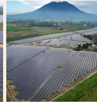
Arayat-Mexico Solar 8 GWh
